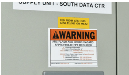
Arc Flash Services and Labeling
