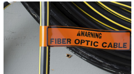
Fiber Optic Cable Markers
