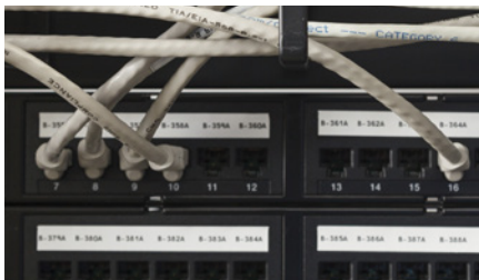
Patch Panel Labels
